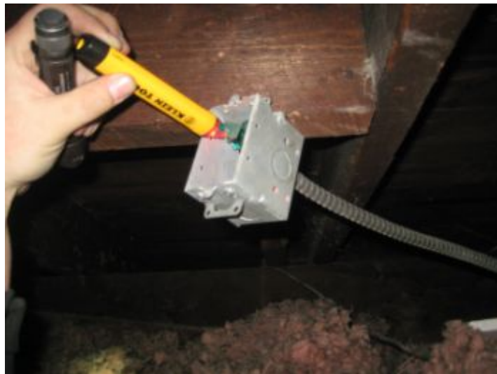
Open junction boxes present in attic with uncapped & charged electrical wiring
