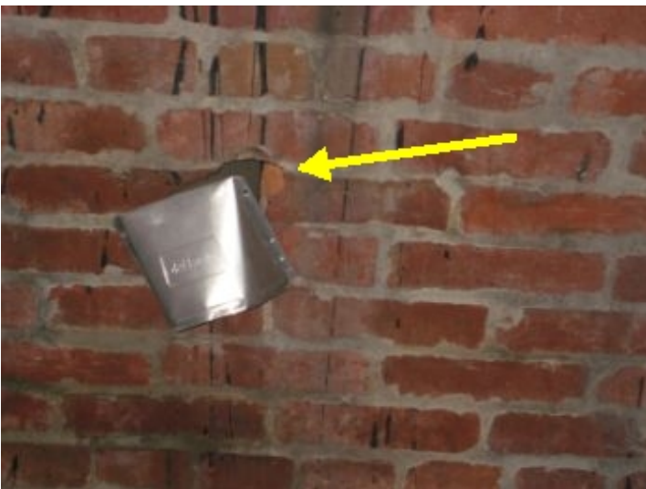
Exhaust fan duct caps were missing or damaged at the exterior
