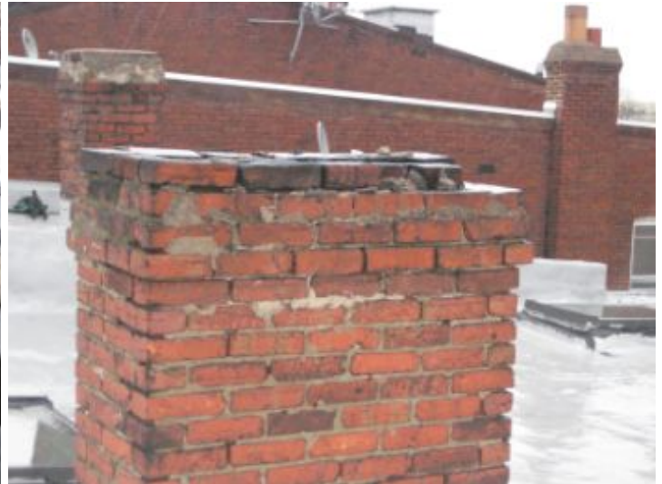
Recommend consulting with a licensed chimney contractor to determine scope of work to repair chimneys & fireplaces
