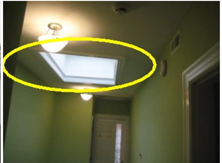
Ceiling around 3rd floor skylight appeared to be damaged from a possible leak
