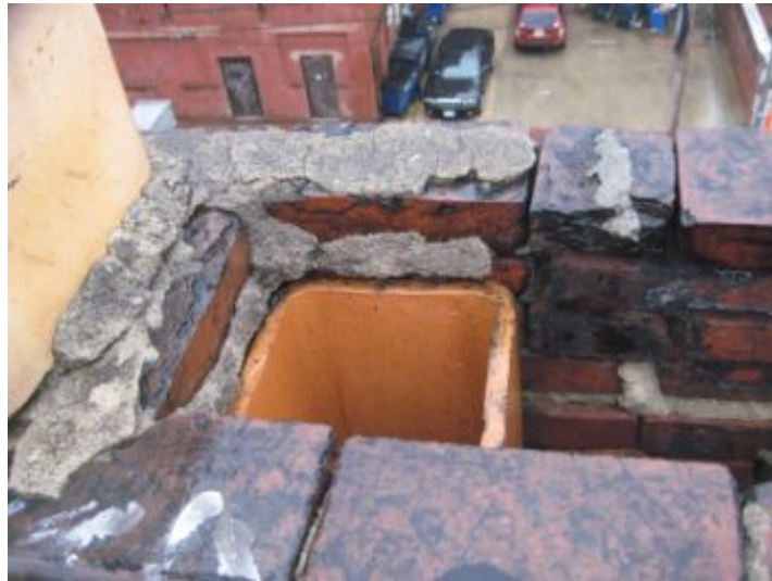
Flues were substantially deteriorated
