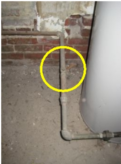
Water heater lacked a working gas shut off valve
