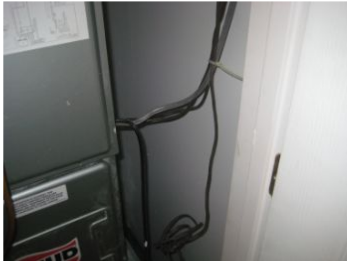
3rd floor AC system lacked an electrical disconnect switch
