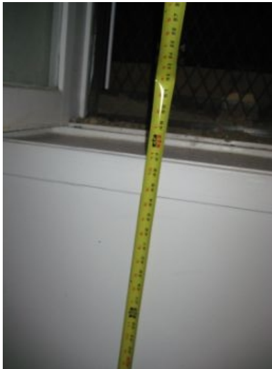
Rear basement window exceeds height requirements for window egress
