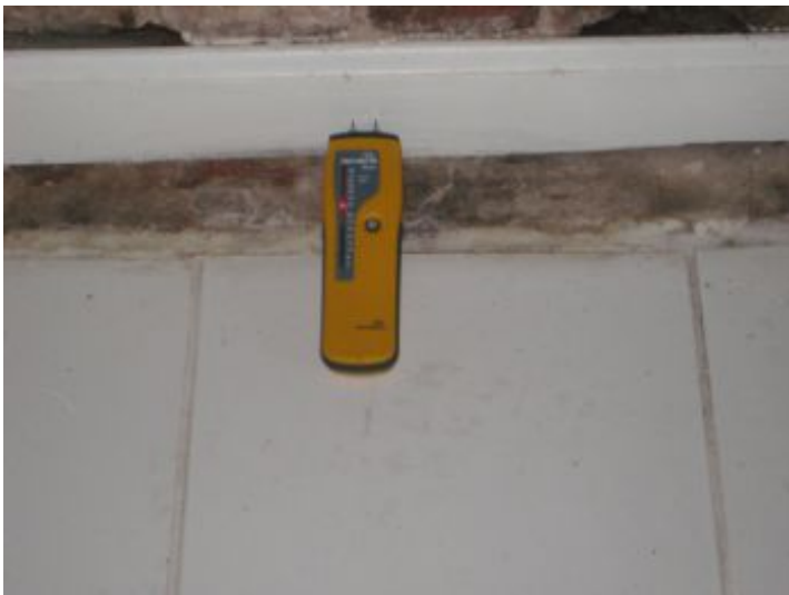
Basement baseboards had an elevated level of moisture present
