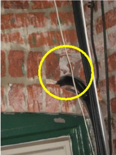
Several gaps present at exterior vent/duct penetrations
