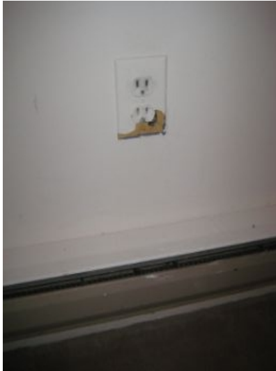
Electrical outlets were located over electric baseboard heaters - fire hazard
