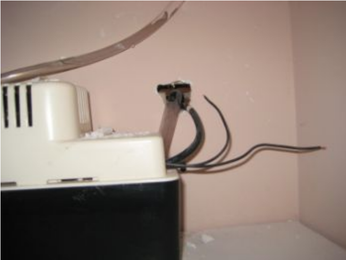
2nd floor condensate pump in plugged into a concealed outlet
