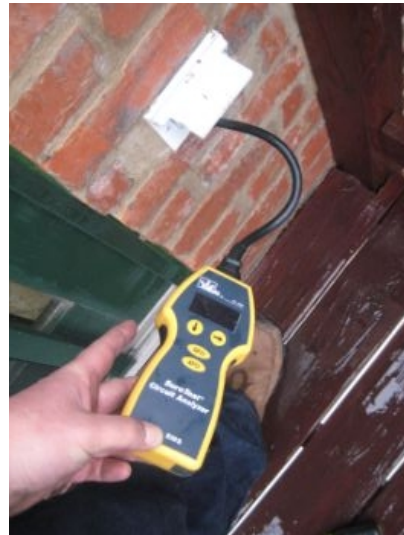
3rd floor balcony GFCI was not working at the time of the inspection
