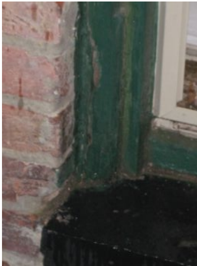
Several rear windows have deteriorated trim and are not sealed against the brick
