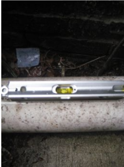
Rear PVC gutter extension did not appear to be negatively sloped for proper drainage
