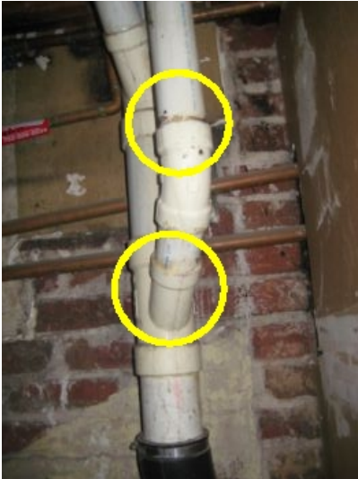
Main drain/waste line in basement mechanical room was leaking at the time of the inspection
