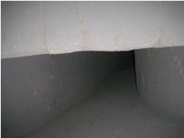
Flues were substantially deteriorated
