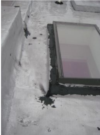
Flashing around sky lights was deteriorated and improperly repaired
