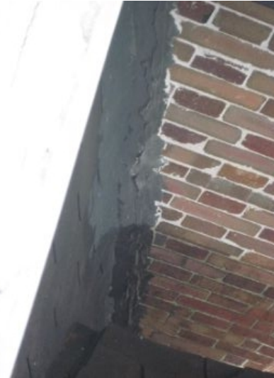
Step flashing at front front was not functional and cover with asphalt based sealant without UV protection
