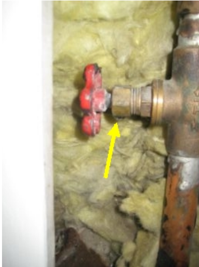
Shut off valve at basement was leaking at the time of the inspection
