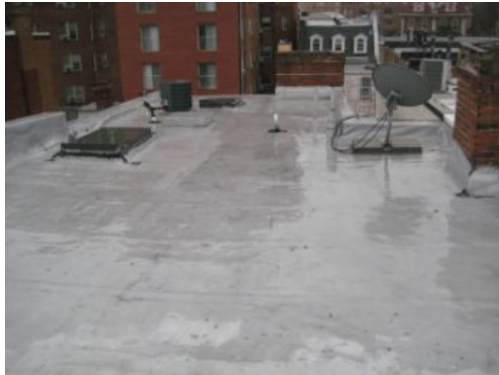
Modified bitumen roof was deteriorated with substantial cracking at the surface
