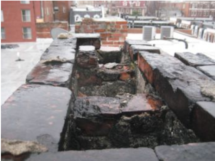
Bricks and mortar were substantially deteriorated at all 3 chimneys
