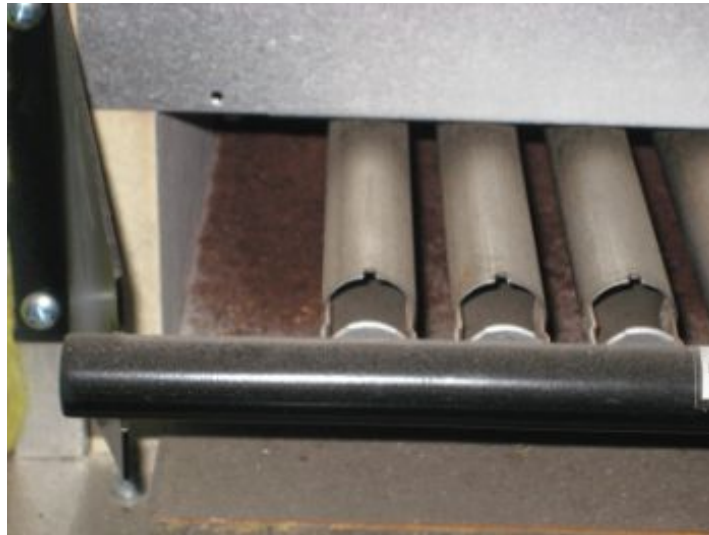
Rust flakes were present in the combustion chamber
