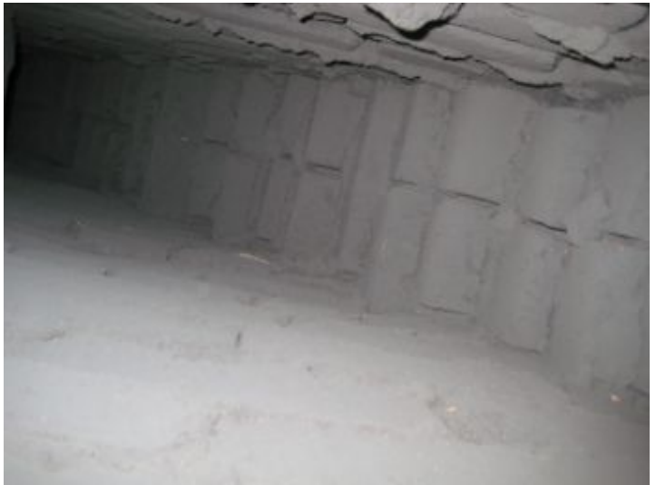
Flues were substantially deteriorated
