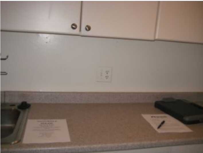
Basement kitchen counter top outlets were not GFCI protected
