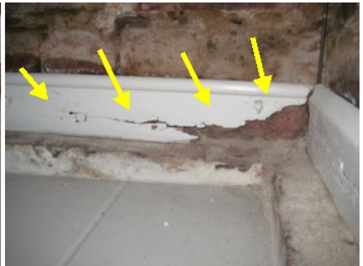
Baseboard at basement floors were substantially deteriorated - possible termite presence
