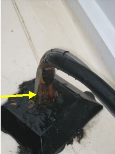
Refrigerant lines at EPDM roof were sealed with expanding foam which was deteriorated at the time of the inspection
