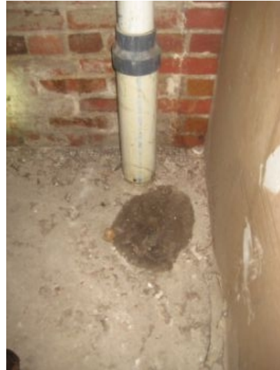
Main drain/waste line in basement mechanical room was leaking at the time of the inspection
