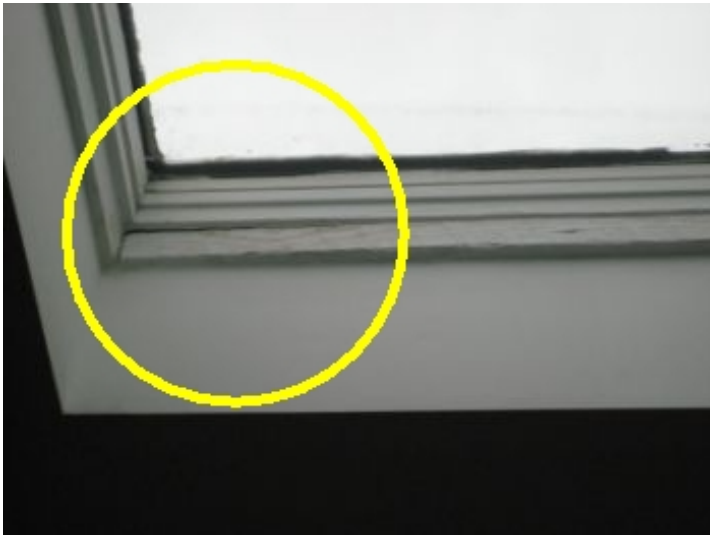
Ceiling around 3rd floor skylight appeared to be damaged from a possible leak
